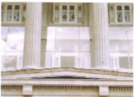
Clever use of plaster for air conditioning ductwork while retaining character of the building
