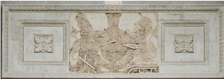
Remnants of damaged crests retained at former Supreme Court
